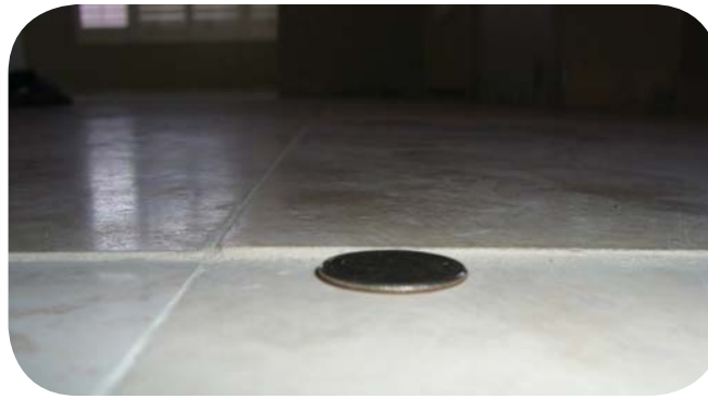
LIPPAGE (UNEVEN TILES)
