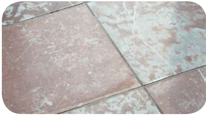
DIRTY, STAINED GROUT LINES
